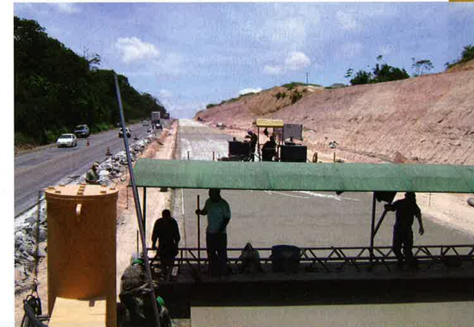
Work being carried out to widen the BR 101 in Brazil, the country's second major highway, and the longest at nearly 4,600km
